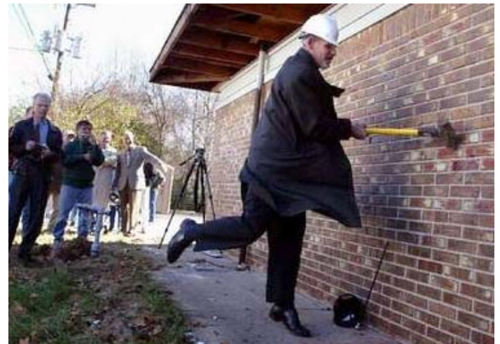
Thomas Cartwright, executive director of The Carter House in Franklin, takes a swing at the former Pizza Hut building on Columbia Avenue as demolition begins.
